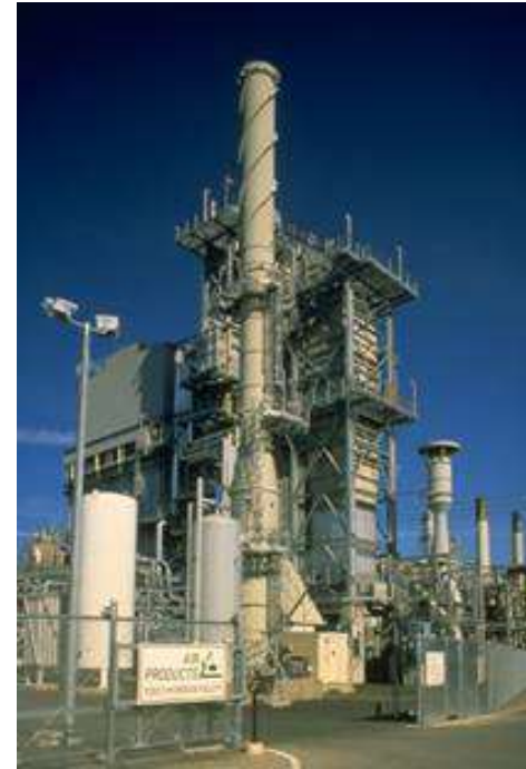
Hydrogen plant in Tosco Corp's Avon refinery 1
