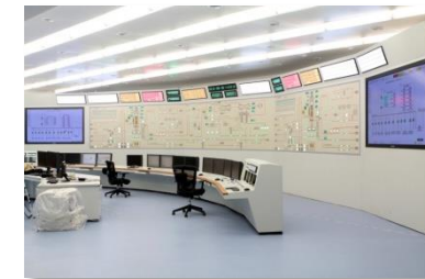
Main Control Room
