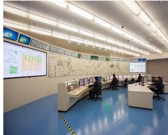
Main control room
