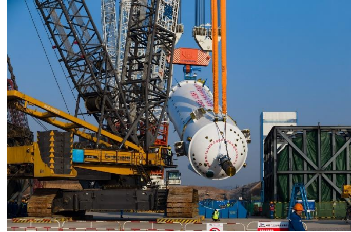
Reactor pressure Vessel
