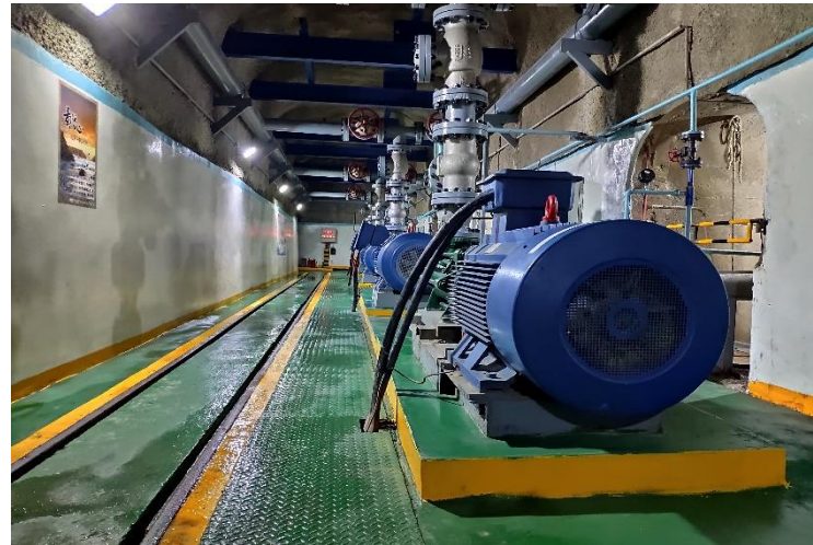
Underground Pump Room Chamber
