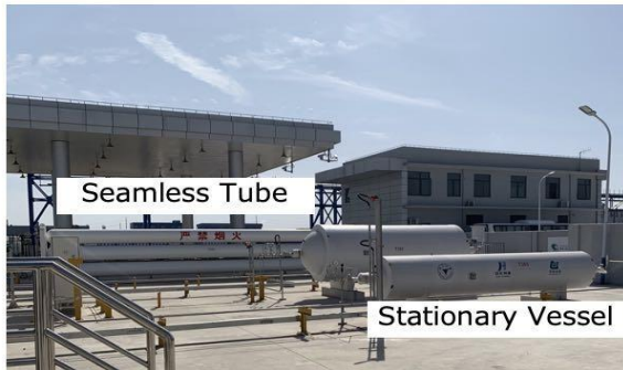
Jinshan HRS, equipped with storage tube and stationary storage vessel
