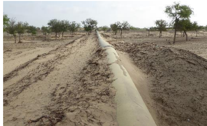
Conveyance system required
